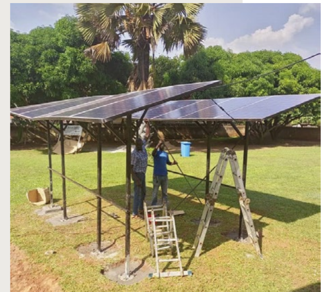
Installation of solar panels at OHCHR in Panama and in Uganda. © OHCHR
